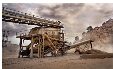
Elastic mesh screen installation for the separation of 7-mm waste rock, with a production rate of 170 ton per hour.
